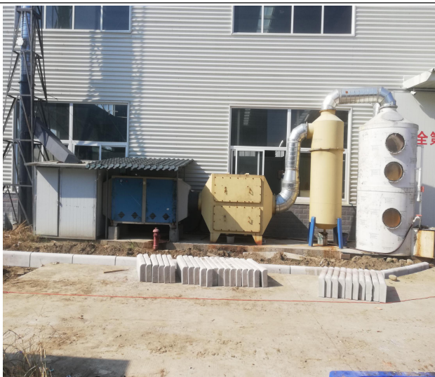
喷淋塔+UV 光解+活性炭吸附箱
